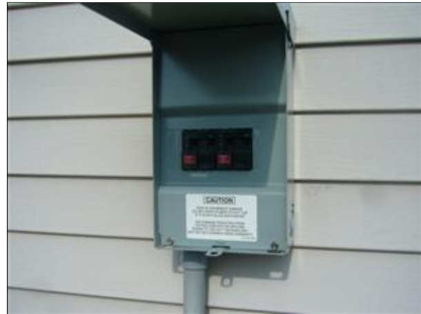
Breaker box for hot tub
