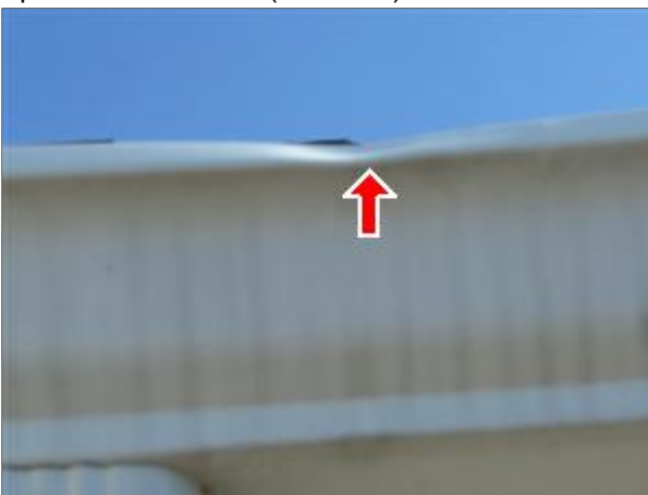
1.4 Picture 1 Left side gutter
