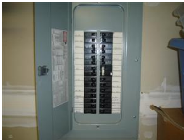
9.7 Picture 2 Main circuit panel
