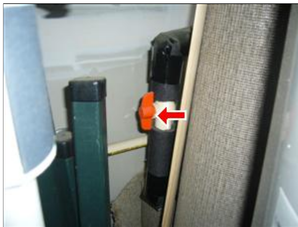
8.3 Picture 2 Inside water shut off
