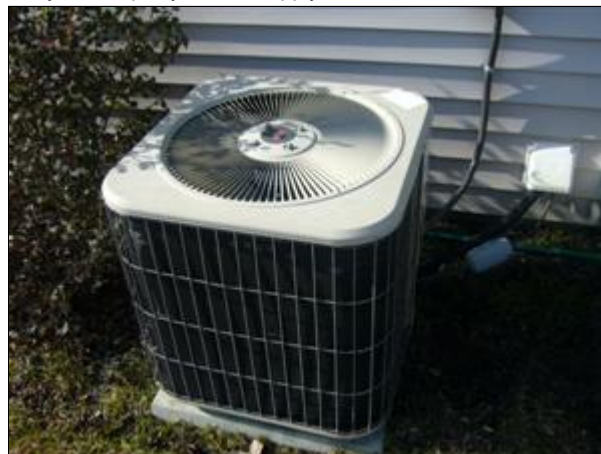
Upstairs cooling unit
