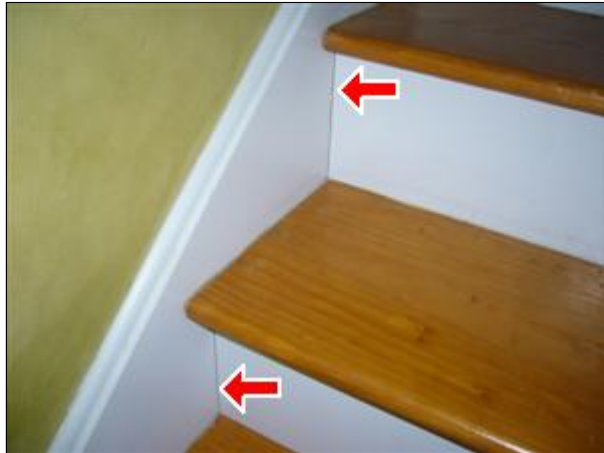
5.3.D Picture 1 Gaps in caulking
