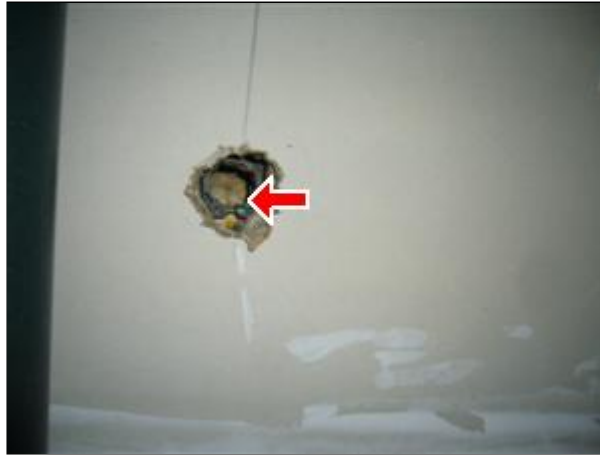
3.1 Picture 1 Hole next to water heater
