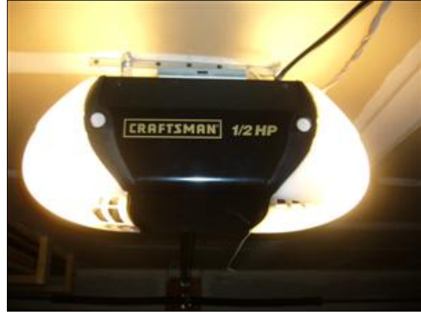
Garage door opener
