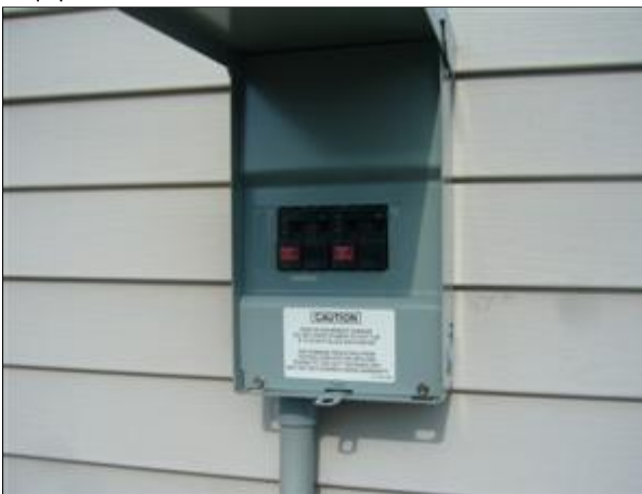
Breaker box for hot tub
