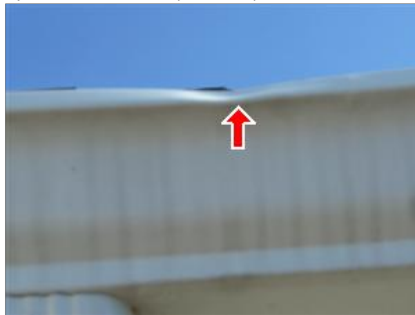
1.4 Picture 1 Left side gutter
