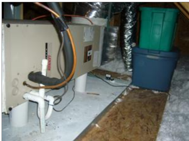
Downstairs heating unit
