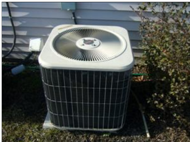
Downstairs cooling unit
