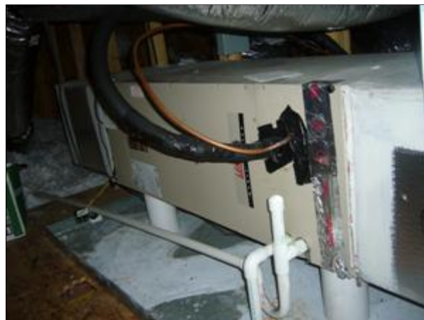
Upstairs heating unit
