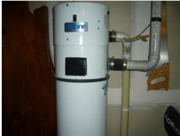
9.10 Picture 1 Vacuum system
