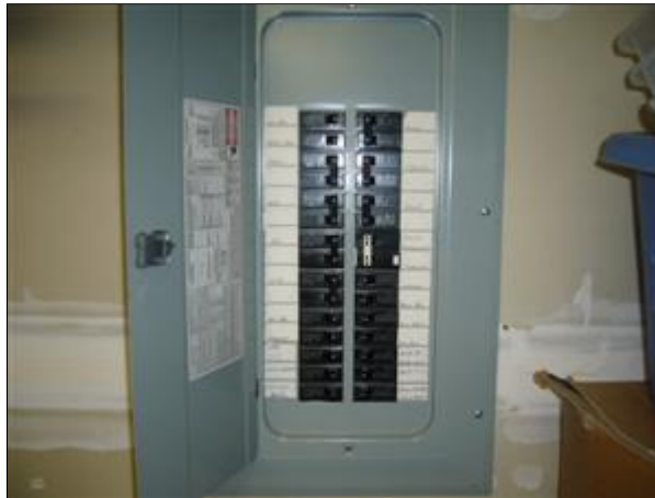
9.7 Picture 2 Main circuit panel
