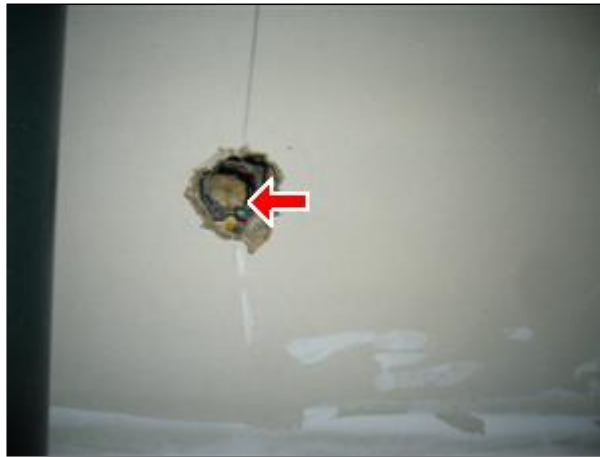
3.1 Picture 1 Hole next to water heater
