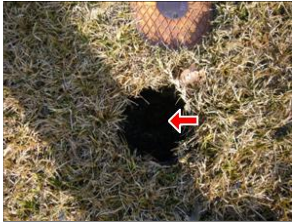
8.3 Picture 1 Main water shut off valve
